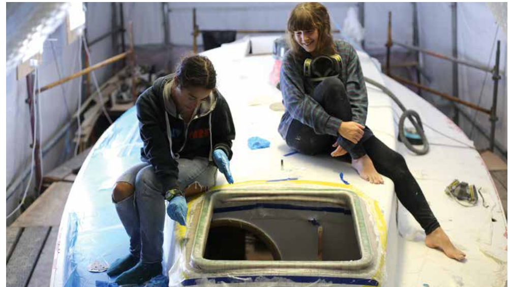
Chloë and Lily glass in a new base for the forward hatch, which had previously leaked. A new hatch is then fitted
