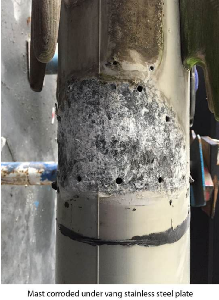
Mast corroded under vang stainless steel plate
